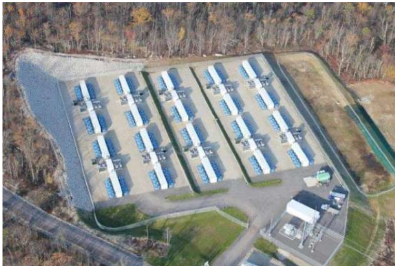
Figure 44: Beacon Power Hazle Township, PA plant 20 MW - 2013
