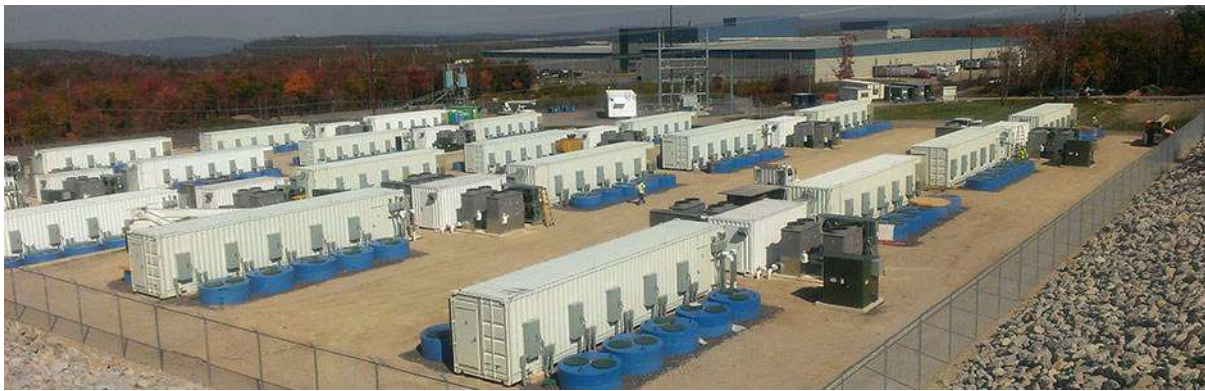
Figure 42: Photo of Beacon Power flywheel installation in commercial operation in PJM, Hazle, Pennsylvania. The plant includes 200 flywheel modules lowered into the ground (5 on each side of a container). The plant currently provides 20 MW of frequency regulation service to PJM and reached full commercial operation in July 2014 [6].
